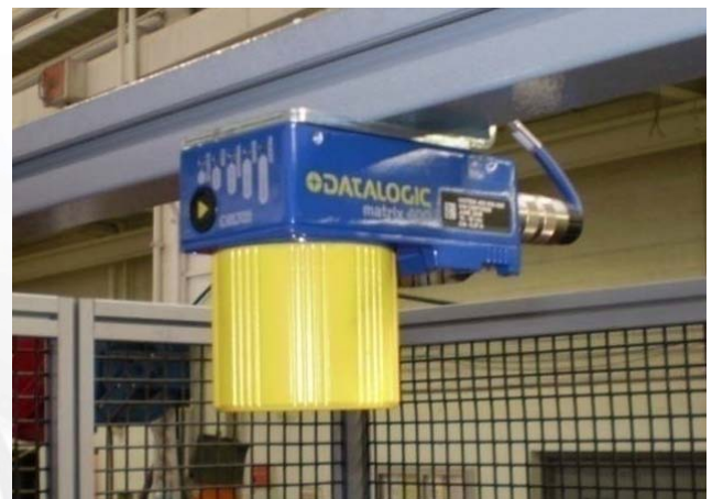
Barcode Reader installed on a tire handler & lube station
